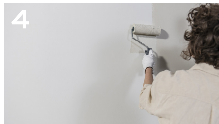
4 Paint your first colour with a roller. This acts as a base layer.
